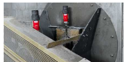
Lubrication of a pillow block bearing on a blower
